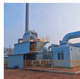
VOC treatment equipment at the Tianjin site
