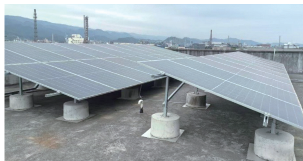
Solar power generation that started in November 2025 at the Chongqing site
