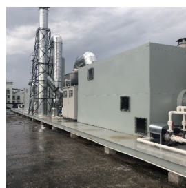
VOC treatment equipment at the Zhongshan site
